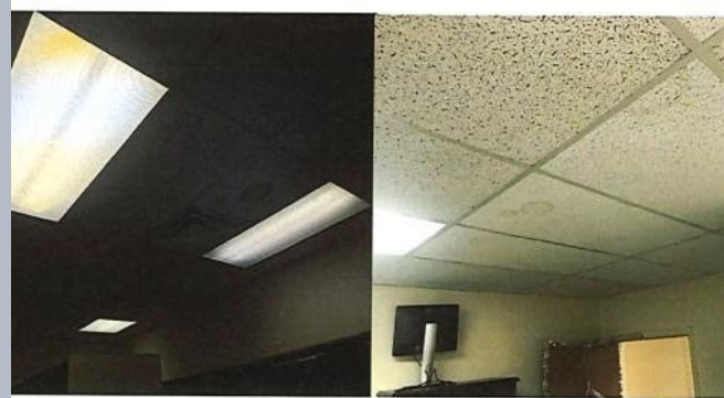
10 - Law Library / Leak shown in Light
