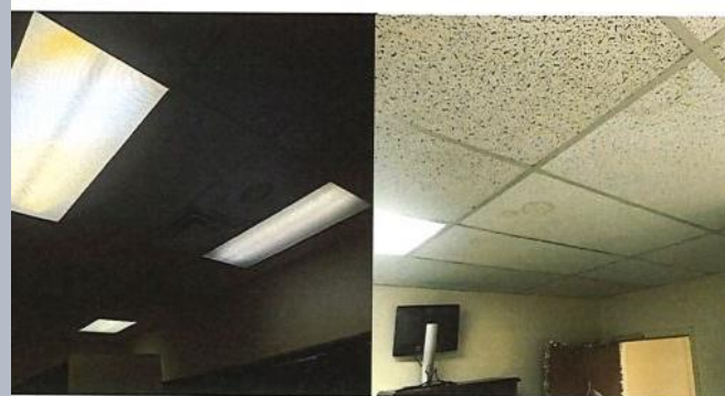
10 - Law Library / Leak shown in Light
