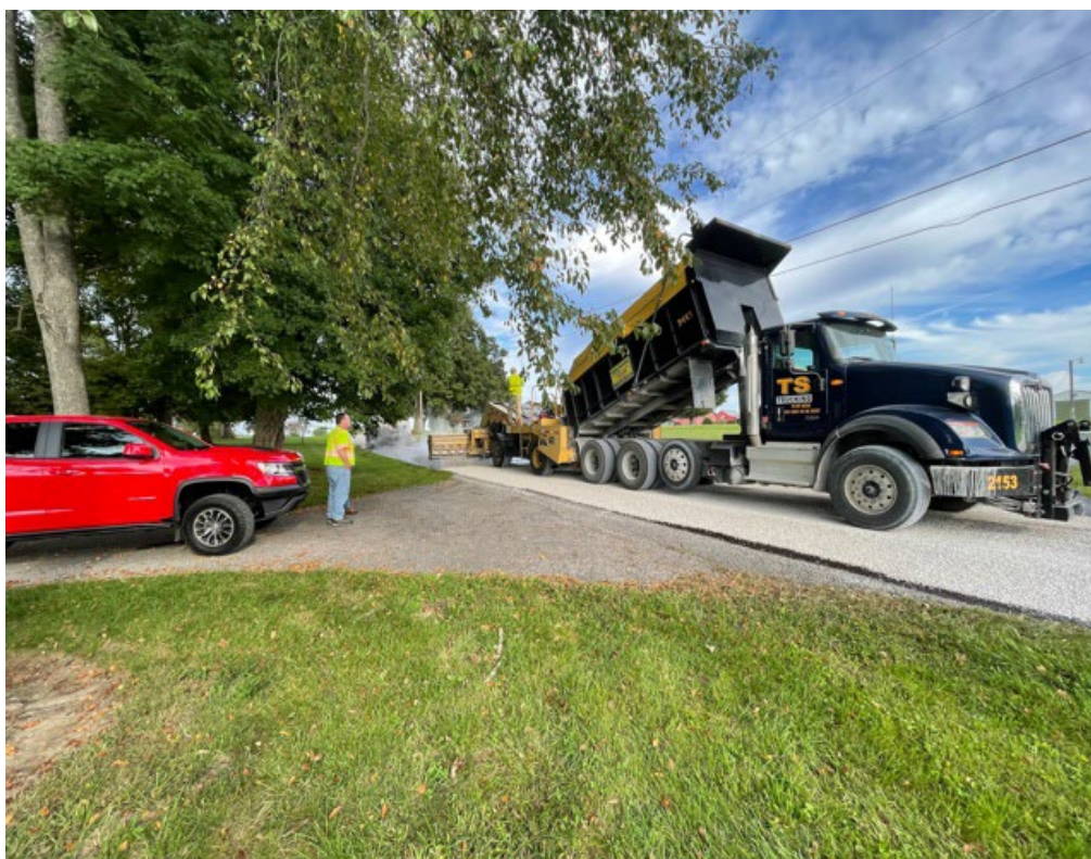
Photo 1. RMA Paving Project, Smith Mill Road, Hardin County Photo by Hardin County Road Department
