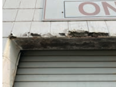
Overhead door lintel, CMU is in a heavy state of deterioration
