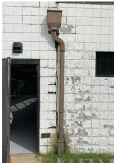
Image retaken September 2020, note CMU has continued to deteriorate.
