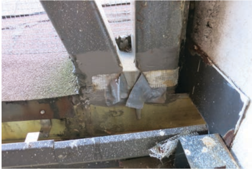
Gutter & through-wall scupper
