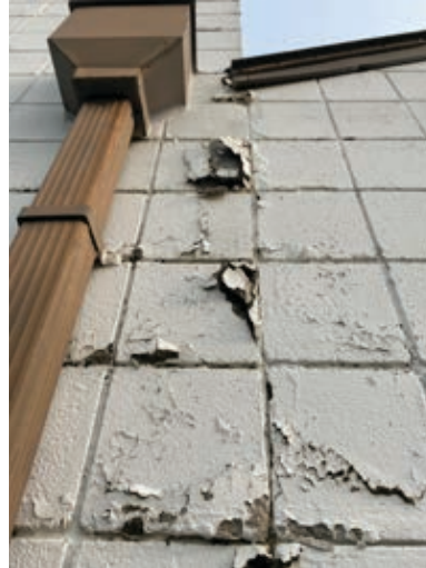
Paint and CMU spald adjacent to through wall conductor head. Typ at most conductor head location, especially along South Facade
