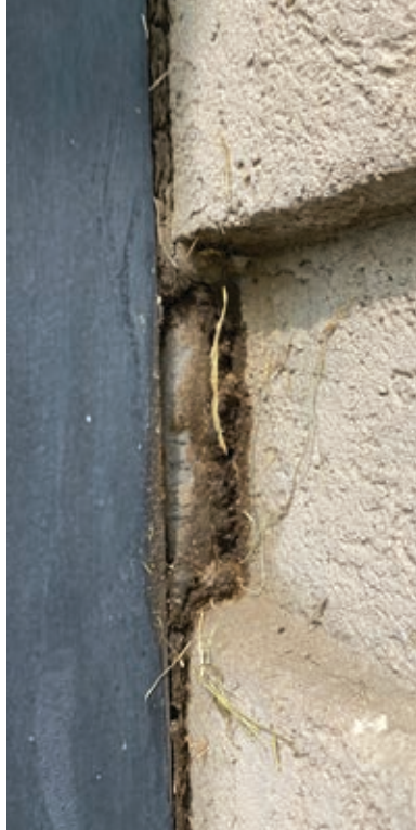
Front entry doors perimeter joint sealants have almost completely disintegrated
