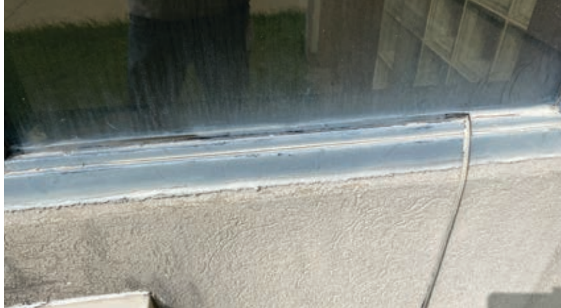
Failed previous repair attempt at hollow metal window
