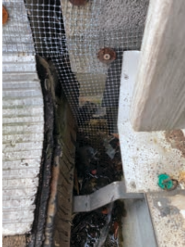
Gutter through-wall opening at expansion joint, which is allowing water infiltration into CMU wall, note joint is completely open on back side
