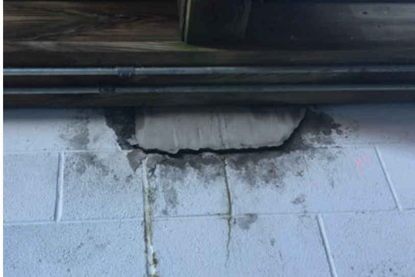
Failing CMU beam pocket repair
