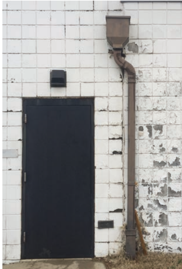
Severe deterioration at control joint
