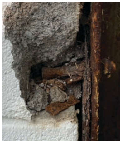
Overhead door track anchors are all heavily corroded and spalling caused adjoining CMU to crack and chip away
