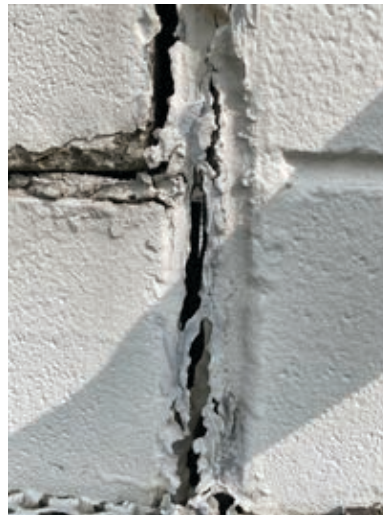
Failed CMU control joint, has opened up allowing moisture infiltration
