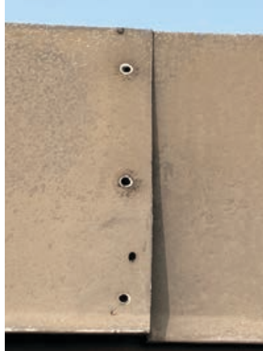
Note pop rivets have failed at top edge of roof flashing
