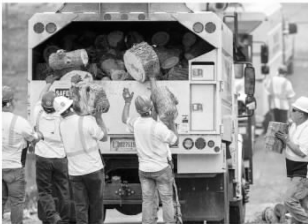
Workers remove sections of trees cut down near the Lansdowne Neighborhood of Lexington on Tuesday.
