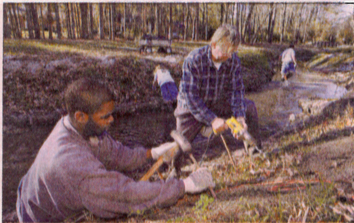
Leon White, right, drills holes for the sticks that LaVelle Walker hammers into place along a section of Hominy Swamp in Wilson. A crew from Coastal Plains Nursery is completing work on a $499,000 Wetlands Restoration Program project that began last summer.
