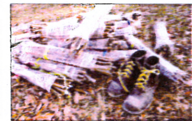
'Live sticks,' which are viable branches from native plants and trees, are planted to restore the banks of eroded waterways. STAFF PHOTO BY HARRY LYNCH
