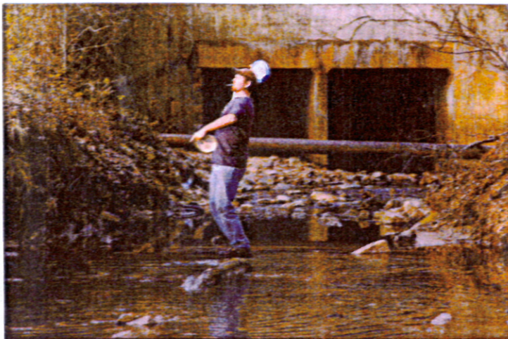
Greg Stahl of Raleigh loses a flying disc after retrieving it from a stream at Kentwood Park. Foot traffic at the park has eroded two streams, which the Wetlands Restoration Program plans to restore at an estimated cost of $540,000. The project has been delayed for two years.
