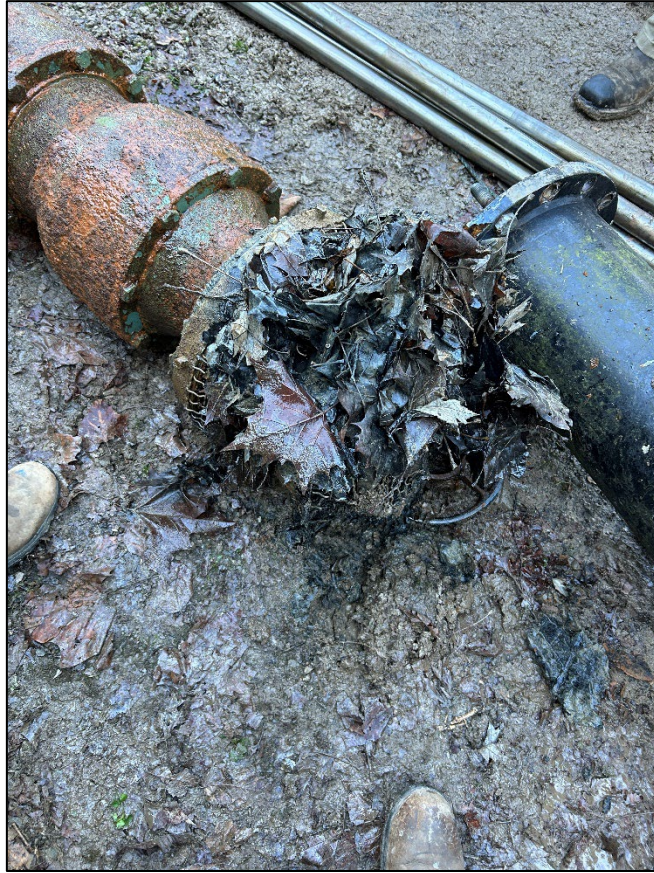
Photo: Inoperable pump pulled from Cynthia Water Works Licking River backup intake
