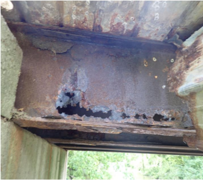
Beam 1, span 2, at Pier 3. There is a ~27" long x 6" high hole that tapers to a 2" high hole, ~7" from the Pier 3 face.
