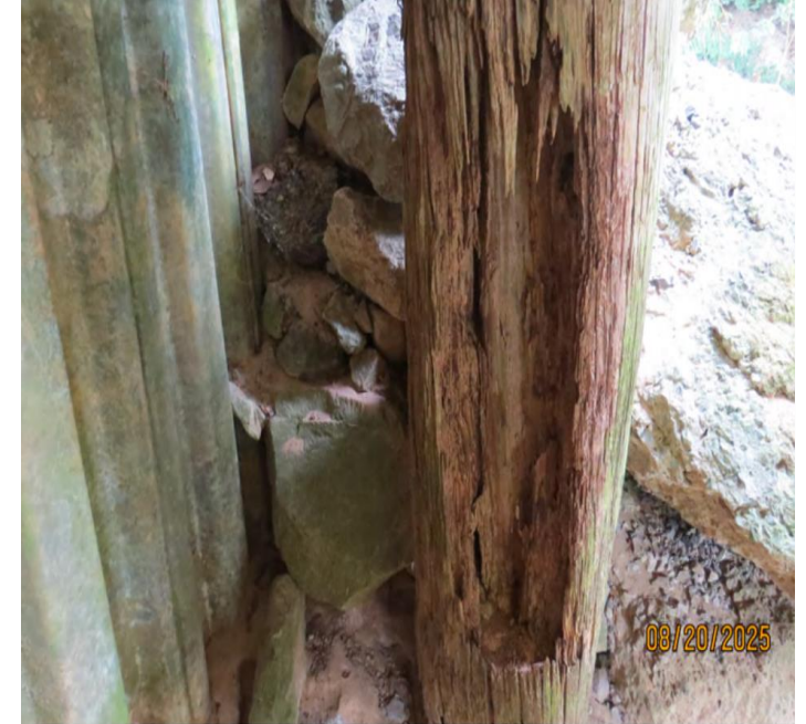
Abutment 1 - pile 1, heavy decay consider failed = CS 4
