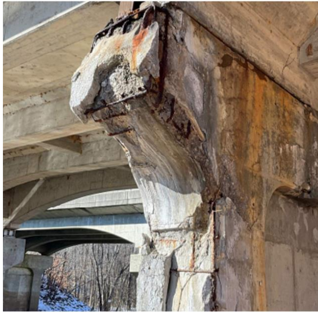
Exposed rebar on Pier 4 right side
