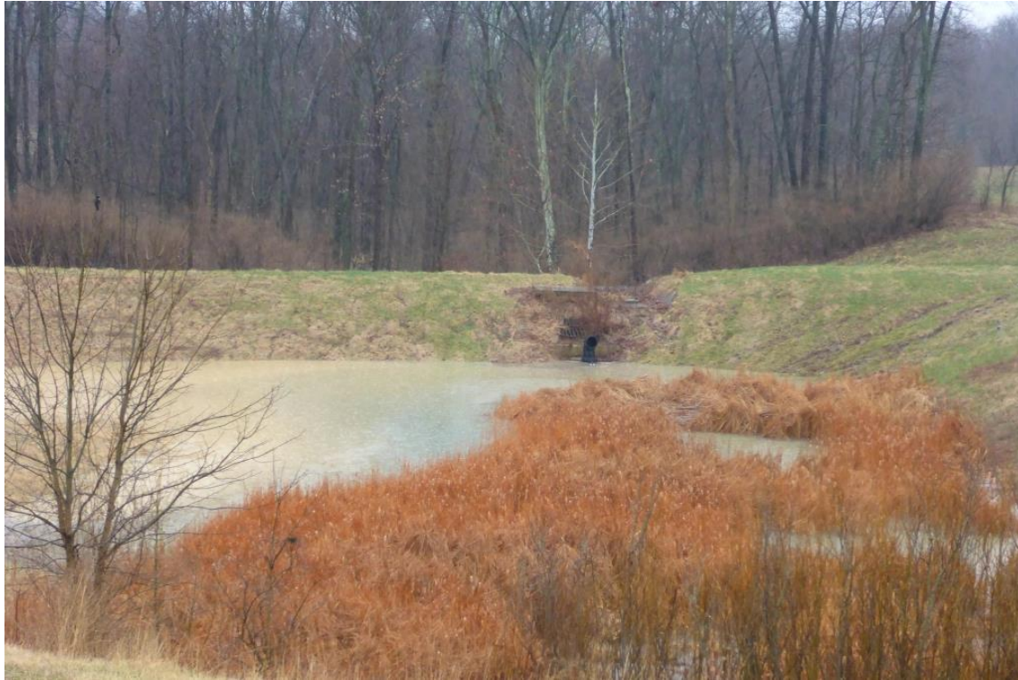
Figure 4: A retrofitted Detain H@) stormwater detention basin. Photo credit: Bob Hawley Source: https://www.flickr.com/photos/govandybeshear
